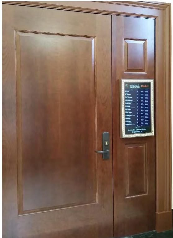
Figure 49. Old Solano Courthouse courtroom door, with electronic sign affixed onto the door.
